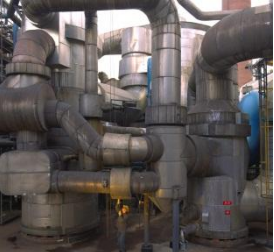
Sulphuric acid plant
